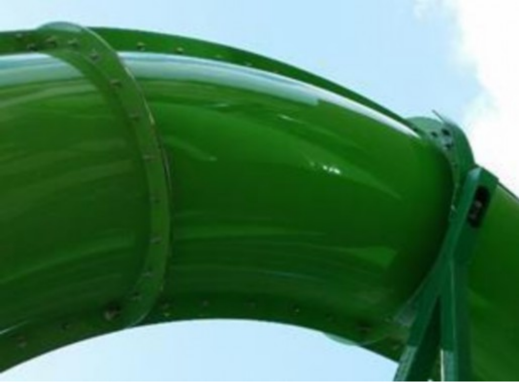
Figure 74: Buffed and Clear Coated Large Repair, Outside
