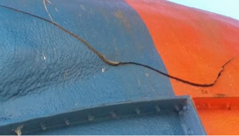
Figure 14: Crack in FRP
