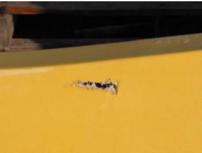
Figure 15: Puncture Holes in FRP
