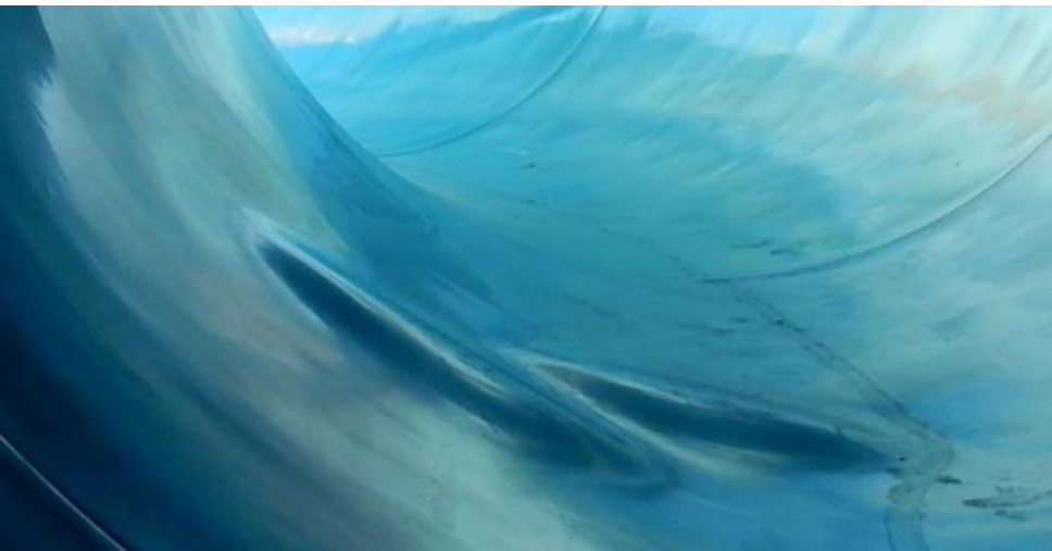
Figure 17: FRP Deformation, Slide Path Obstruction
